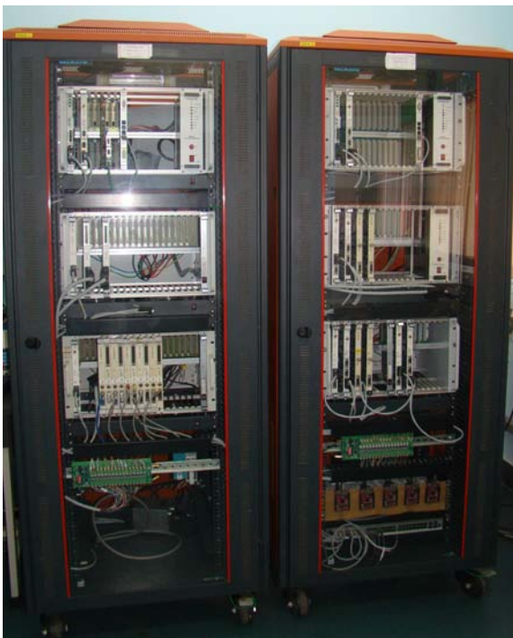
Fig. A.3.1: VME racks with L-2 and L-3 stations.
