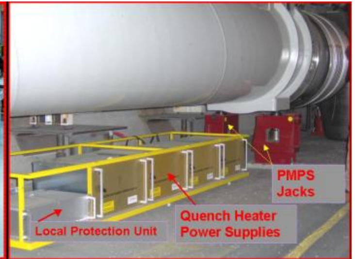
A part of DAE's contributions 2 installed in LHC Tunnel at CERN
