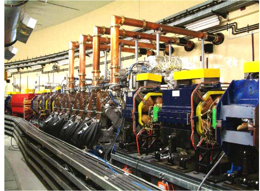
RF Cavities installed in Indus-2 Ring
