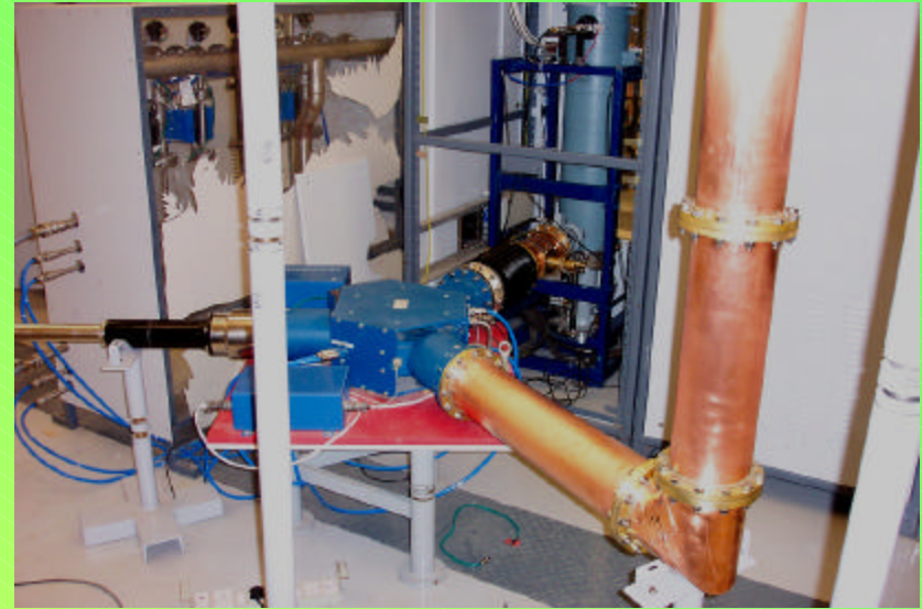
Co-axial Line, Circulator & Klystron
