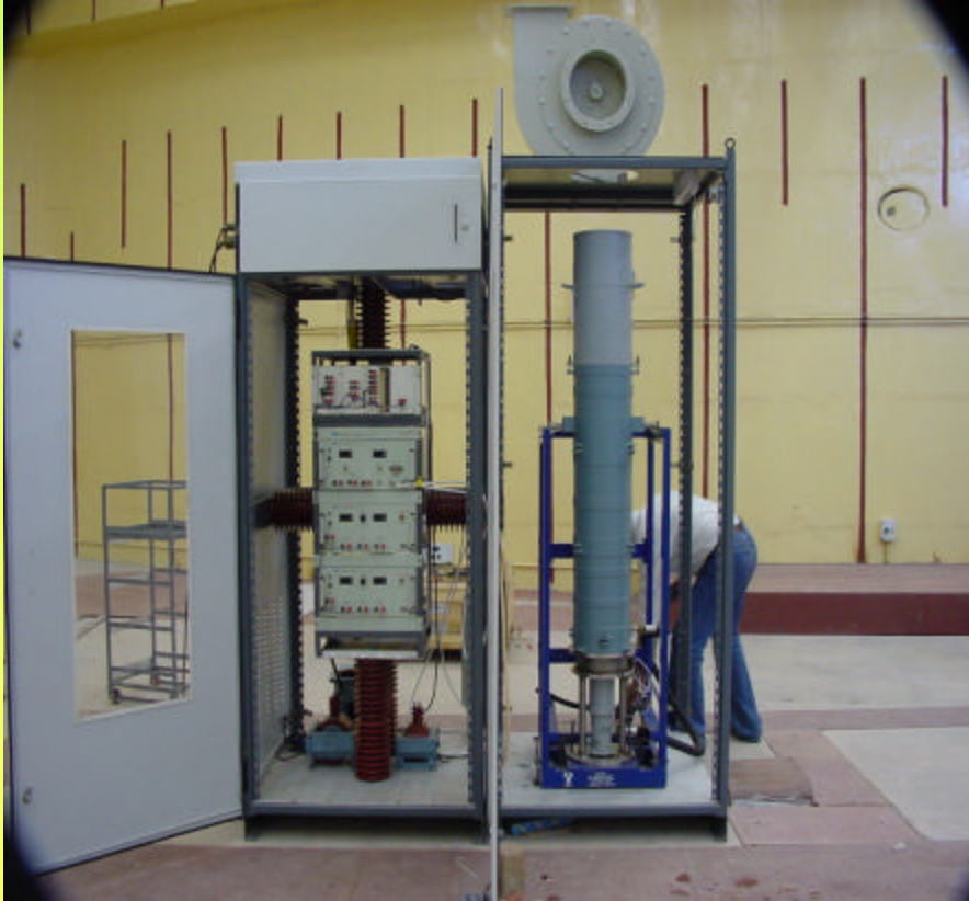
Klystron Tube & Auxiliary PS / Interlock
