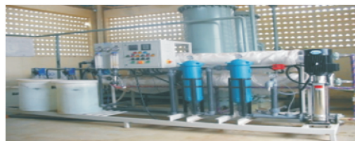
Fig. I.4.2: Reverse osmosis plant.
