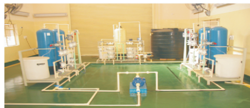
Fig. I.4.3: Ion exchange plant for zero discharge.
