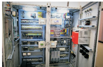
Fig. I.5.2: View of the control panel.
