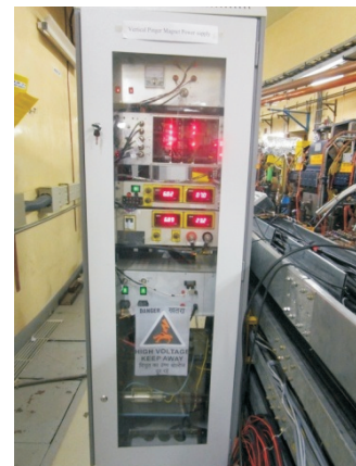
Fig. A.4.4: Photograph of the power supply commissioned in Indus-2.
