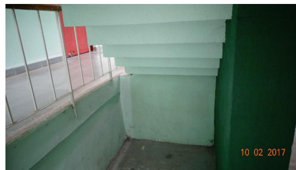
Under the Stairs of R&D Block-A after the SEVA
