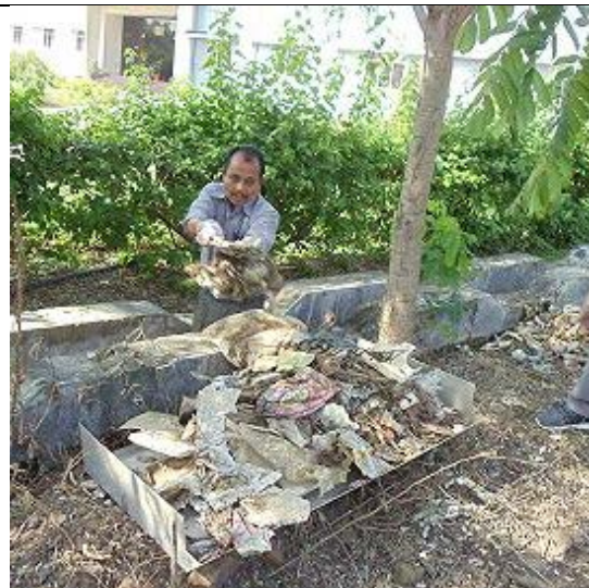
Picking up the poly-bags thermocol pieces and mud deposit from the drainage trench (North side)
