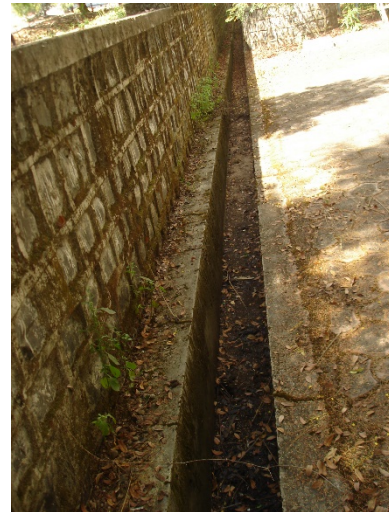
Cleaned drain outside FEL complex
