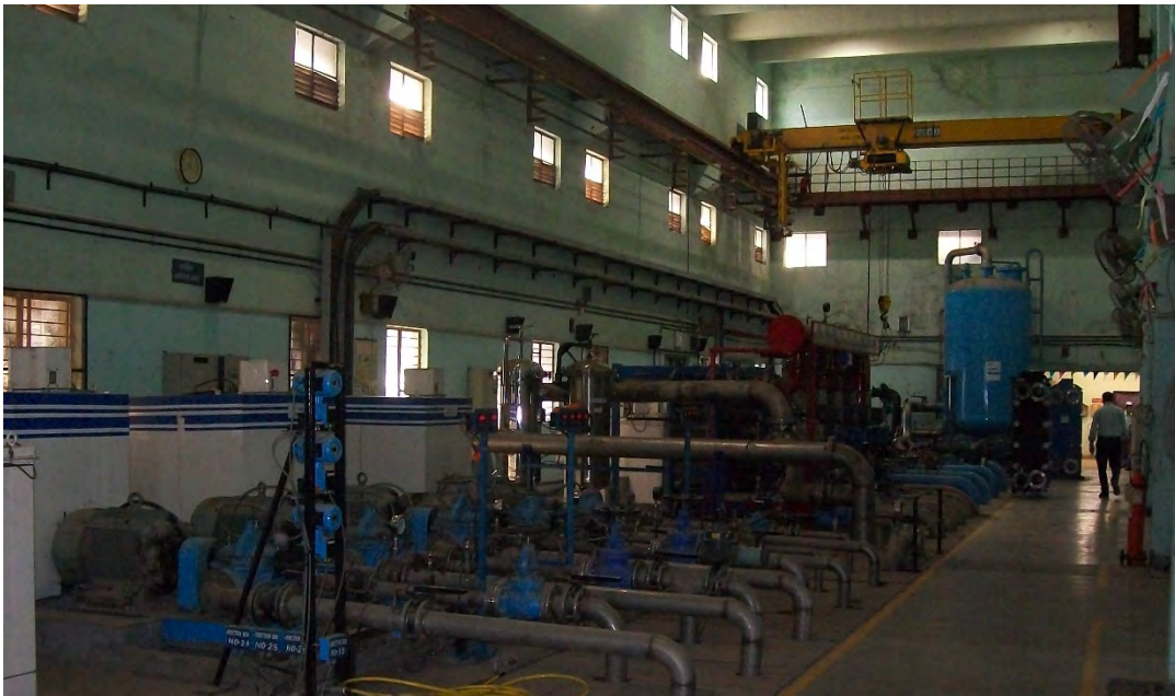
Indus-2 LCW Plant Area along with equipment
