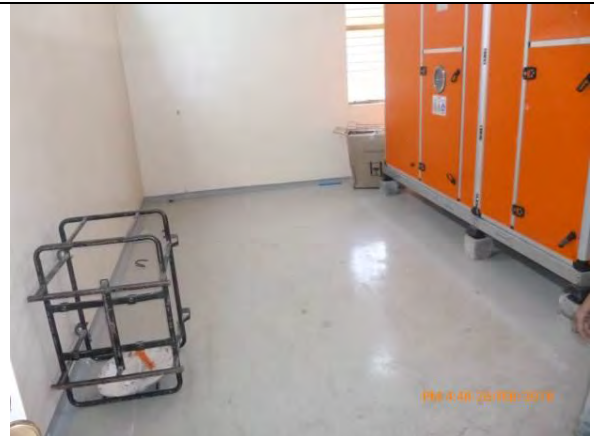
AHU Room (After)
