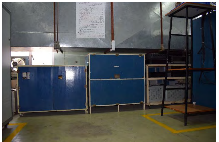
LPSD: D 6BLOCK, ROOM NO. 117, LASER POWER SUPPLY HALL (PARTITION-3)
