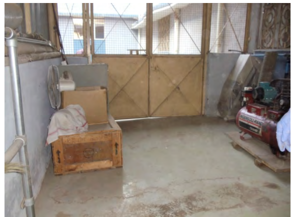
EBW Chiller Shed after cleanliness' drive (SCRF Building)
