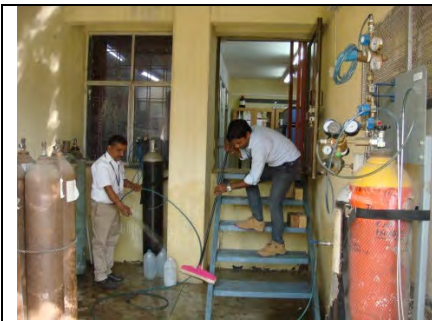
Gas storage area of CO 2 laser lab
