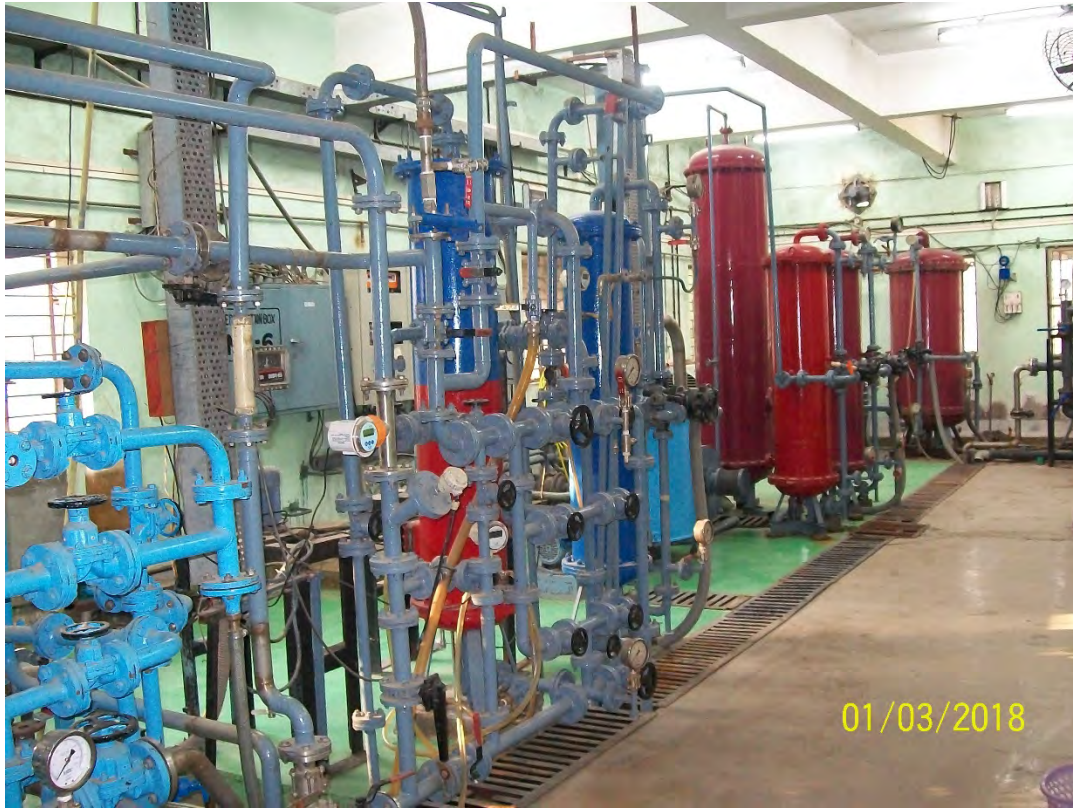
Indus-2 LCW Plant Water Treatment Area
