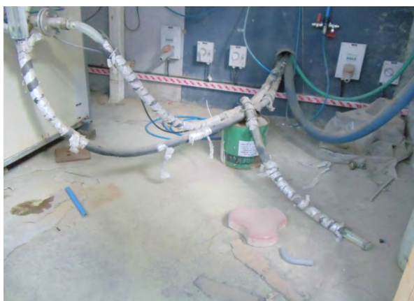
EBW Water chiller piping Area before
