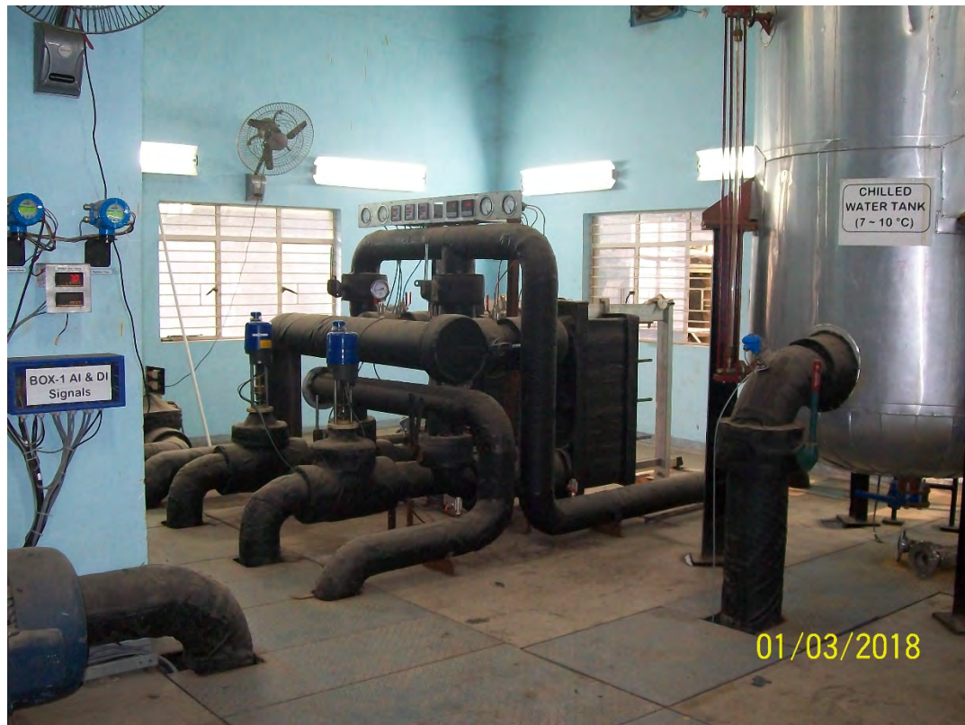
Indus-2 Chiller Building Plant Area
