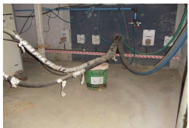
EBW water Chiller after cleanliness' drive
