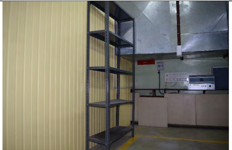
LPSD: D 6BLOCK, ROOM NO. 117, LASER POWER SUPPLY HALL (PARTITION-2)
