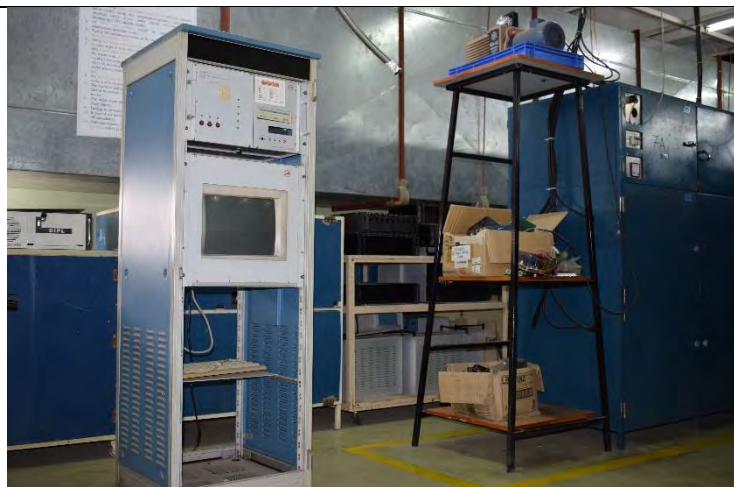
LPSD: D 6BLOCK, ROOM NO. 117, LASER POWER SUPPLY HALL (PARTITION-3)
