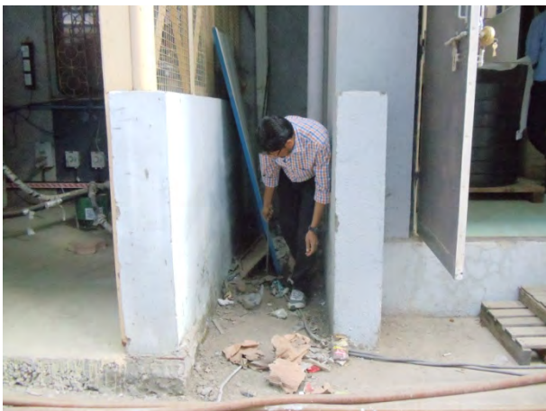
SCRF Building EBW chiller beside area before
