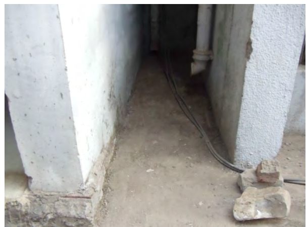
SCRF Building EBW chiller area after cleanliness drive
