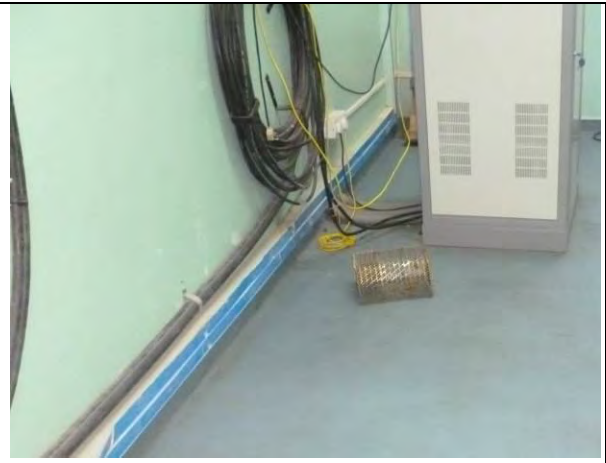
H- building hub room (After)
