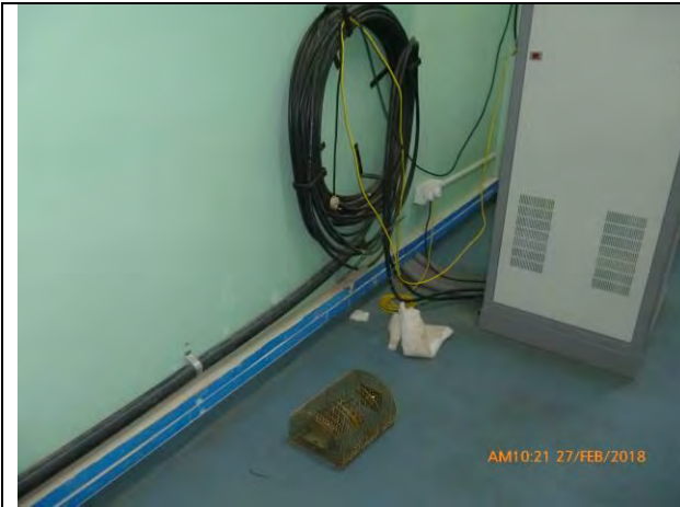
H- building hub room (Before)
