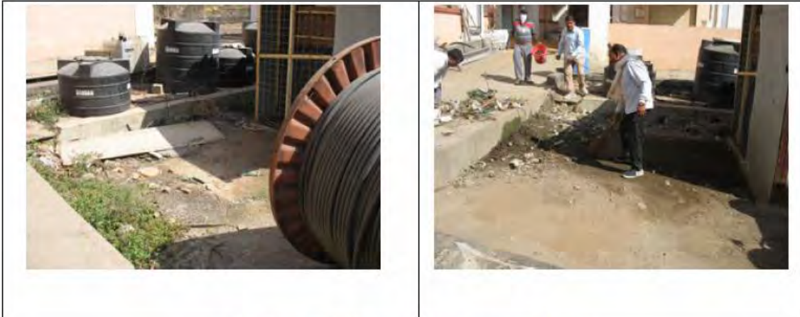
Cleaning by CTF team near compressor room
